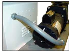
5) Route the other end of the conduit through an empty knock-out and secure with lock-nut. The cord inside will route up to the terminal strip inside the upper portion of the enclosure.
